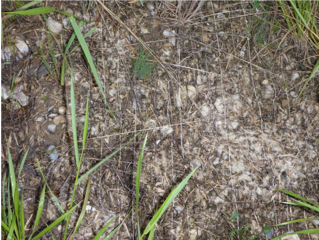
Figure 21: Close-up of the 100% wool ECBs deployed on test slope at Transcend, June 2017.
